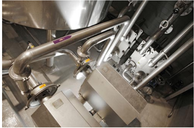
Return pumps and heat exchangers for tank cleaning play the key role in the CIP station.
