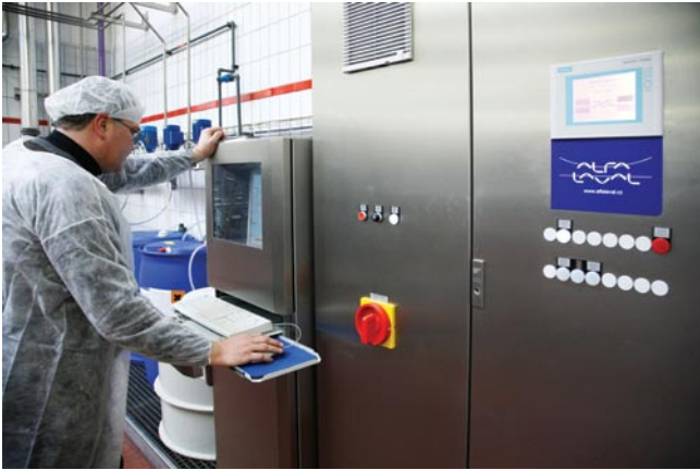
Control of the CIP process is fully automated.
