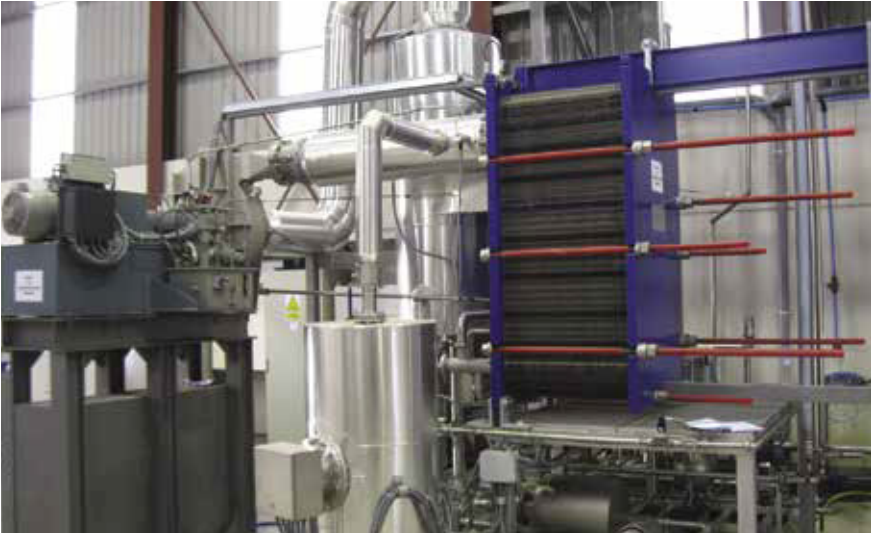
Mechanical vapour recompression system to concentrate effluent. Steam consumption reduced to zero.
