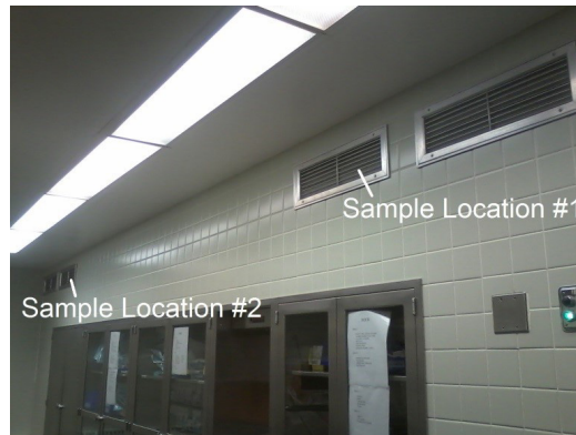
OR Supply Air Diffusers
