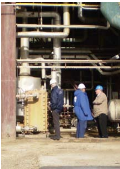
A Compabloc heat exchanger for preheating of Nitric acid
