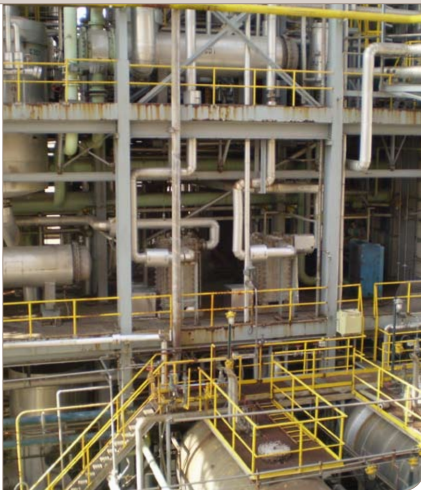
Two Compablocs serving as ammonium nitrate interchangers in the evaporation section of the ammonium nitrate plant. The result? Substantial energy savings
