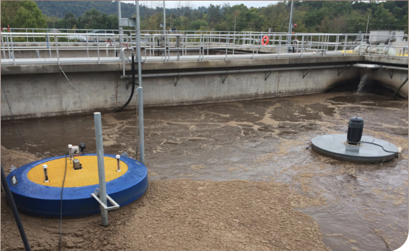
The patented floating decanter in the Alfa Laval AS-H Sequencing Batch Reactor System provides precise decanting for optimum effluent quality
