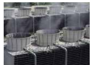
... cooling towers, irrigation etc.
