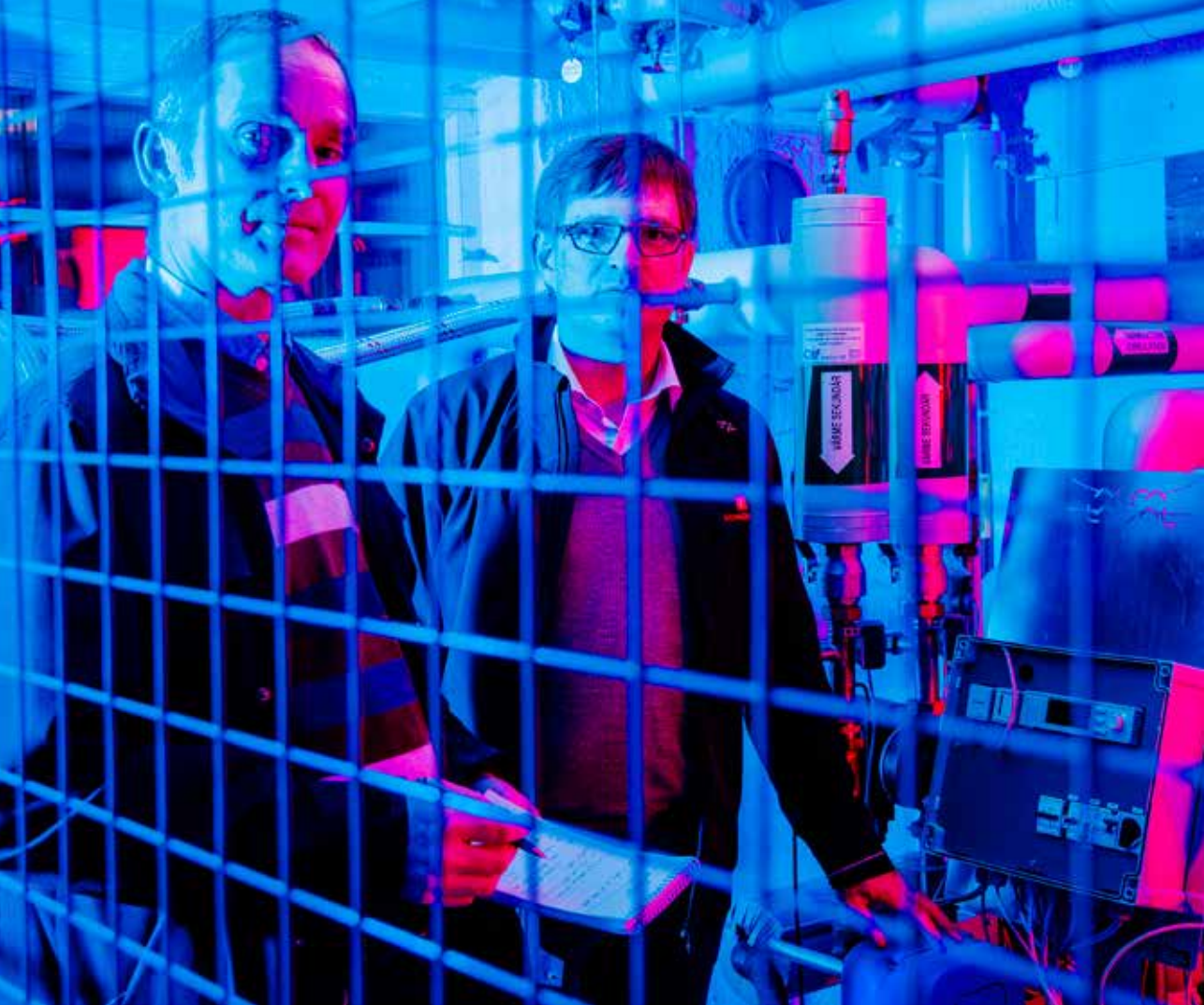
Alfa Laval's Mats Persson, left, and Kristian Olsér, Ronnebyhus' operations chief, in the basement of an apartment block. The total energy savings have been nearly 50 percent.
