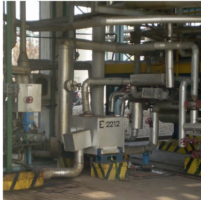
A Compabloc heat exchanger serving as Cyclohexane preheater.
