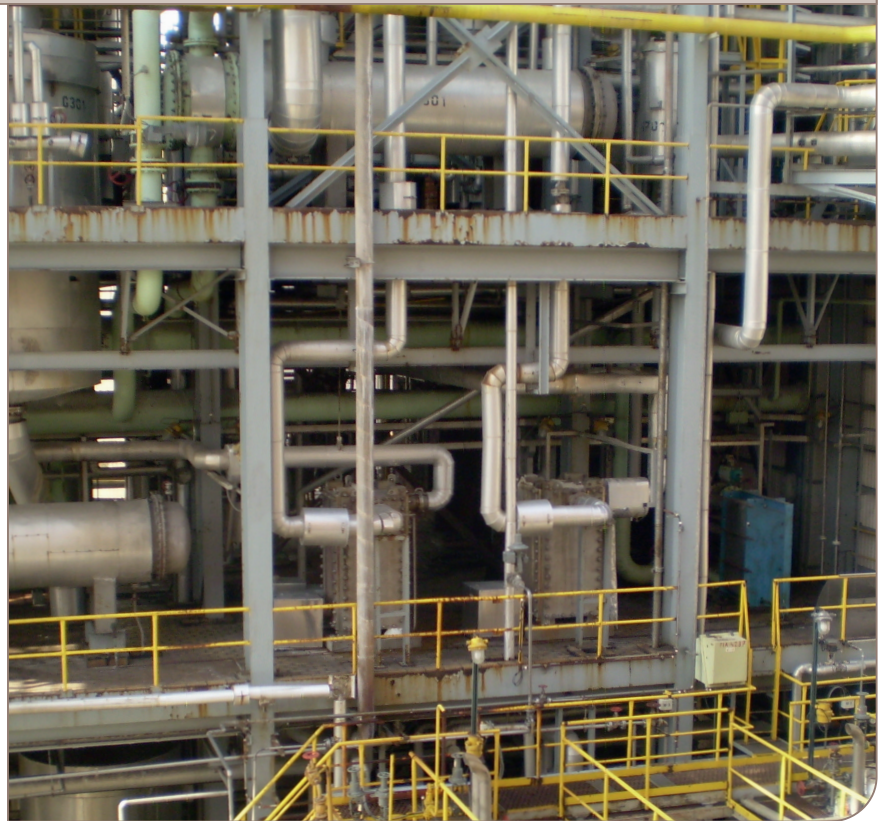
Two Compablocs serving as ammonium nitrate interchangers in the evaporation section of the ammonium nitrate plant. The result? Substantial energy savings
