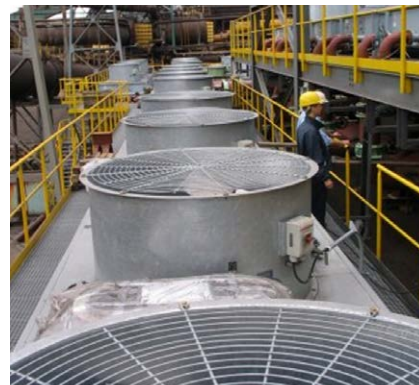
Alfa Laval air coolers at Arcelor Mittal Ostrava
