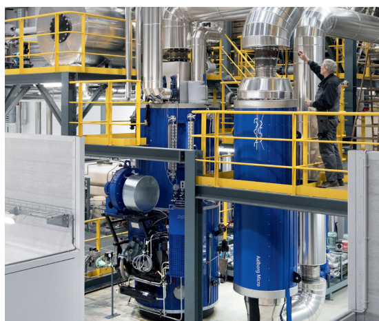
Multi-fuel Aalborg boiler at the Alfa Laval Test & Training Centre
