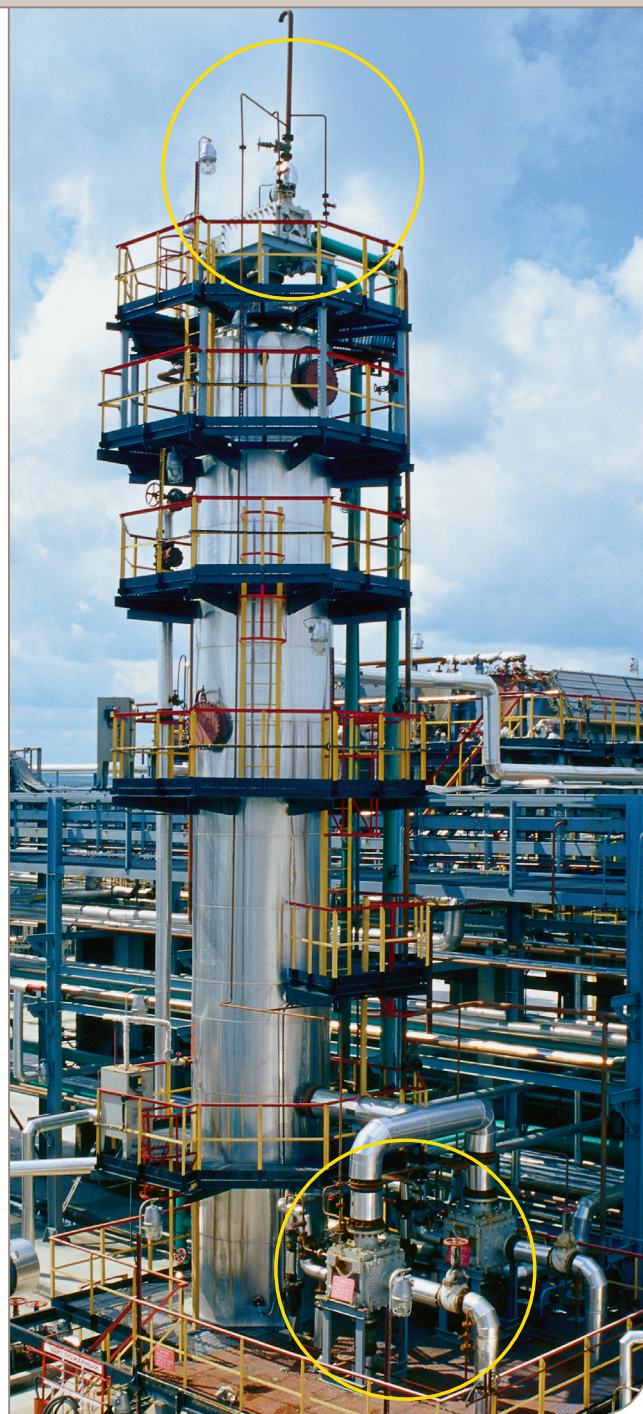
Stripper tower in gas sweetening process, with reboilers and reflux condenser marked with circles (close-ups on next page)
