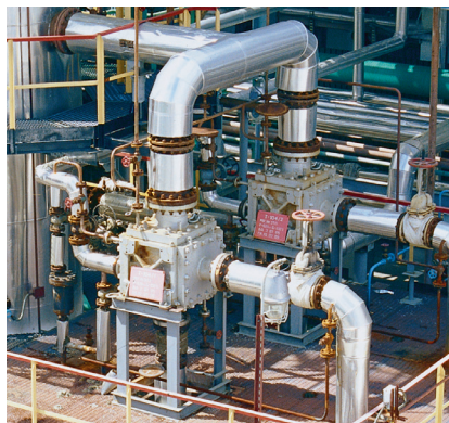
Compabloc reboilers operating with steam as heating medium
