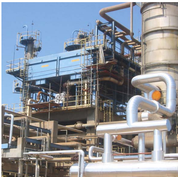
Figure 3. The compact heat exchanger installed just below the primary condenser in the same space used for the old shell-and-tube.
