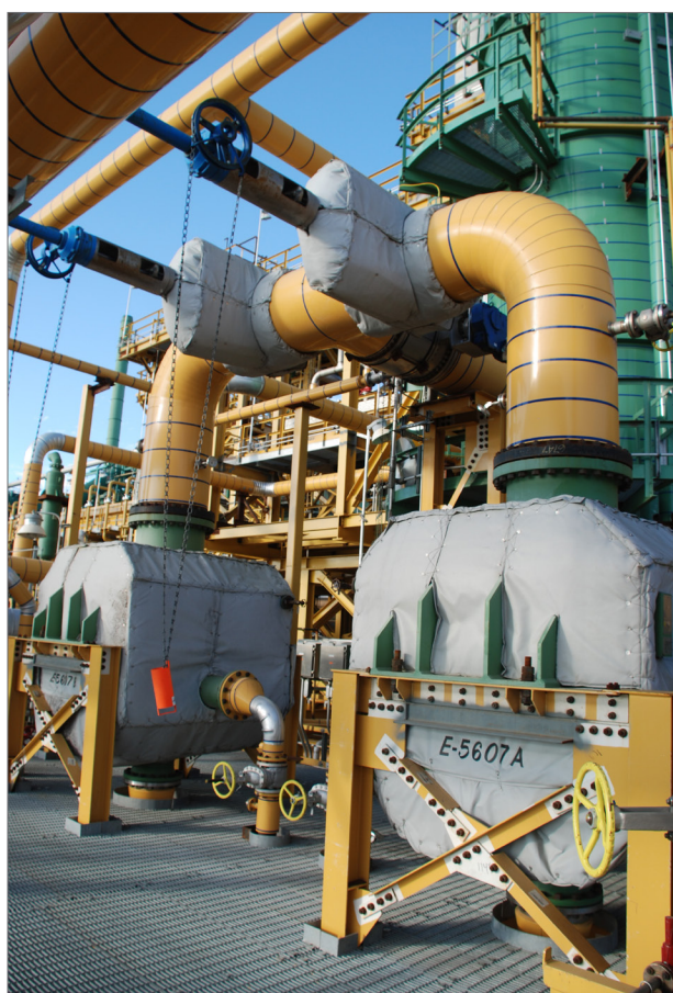
Figure 3 Compabloc reboilers operating in an FCC flue gas treatment plant
